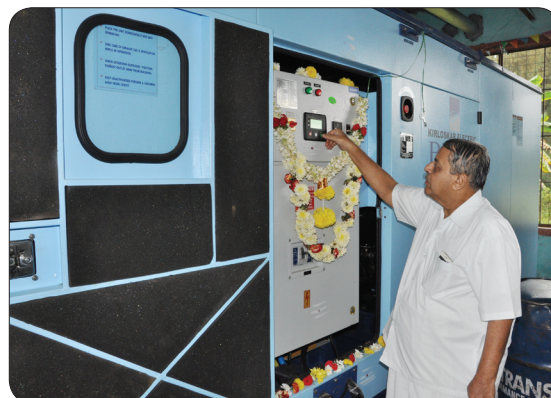
Prashanti Kutiram: Chancellor, Dr. H R Nagendra dedicated a new Generator
